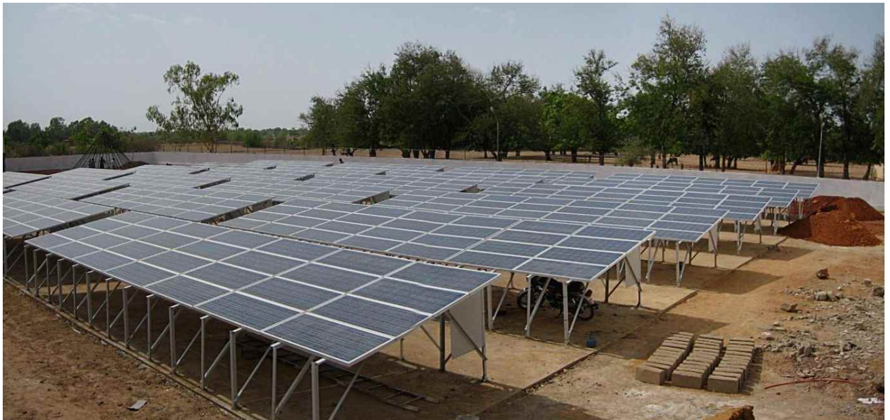
The Fres solar array with in total 72 kWp of solar modules
