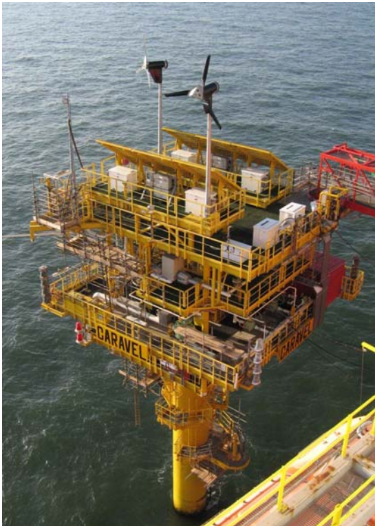
Hybrid solar-wind system offshore on Caravel platform
